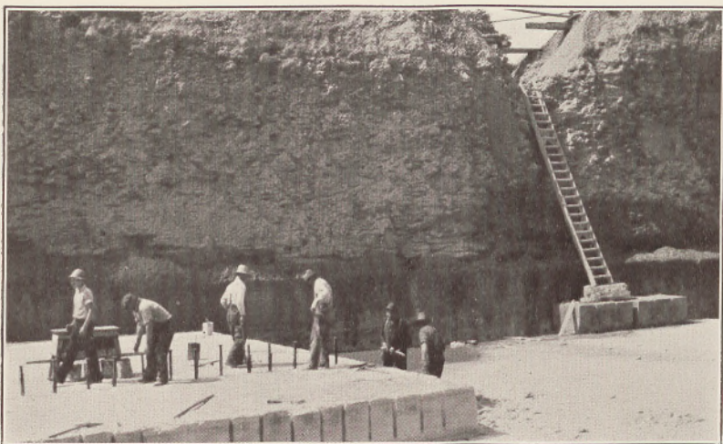
B. WEDGE AND FEATHER SYSTEM OF BREAKING SANDSTONE BLOCKS IN QUARRY AT BEREA
