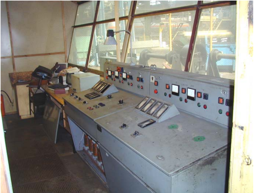
Fig. 3. The control room
