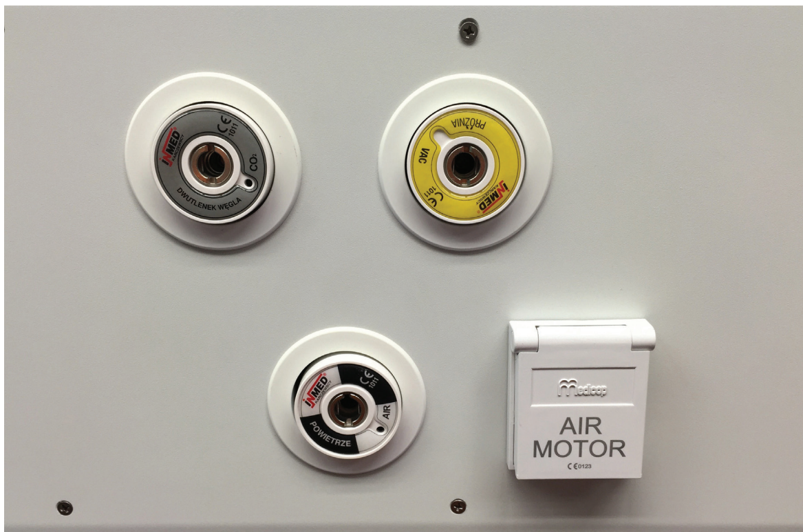
Photograph 6.2.3 Terminal units for medical gas pipeline systems (technical infrastructure may become a hospital-acquired infection source); photographed by the Author, 2016
