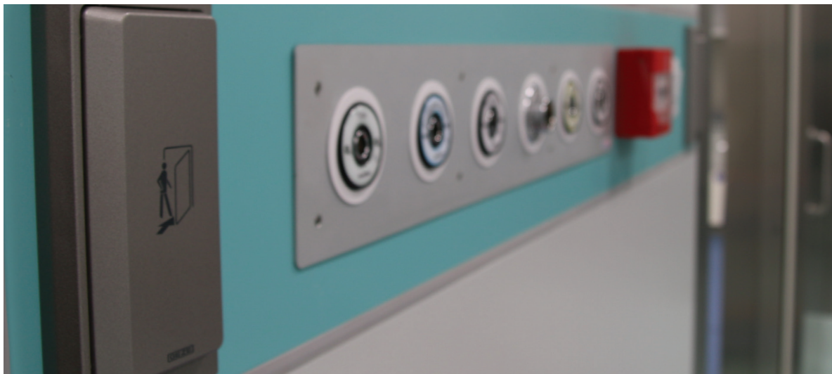
Photograph 5.5 Elements of wall finishing at an operating theatre (an example of a surface characterised by an increased resistance to disinfection procedures); designed and photographed by the Author, 2016
