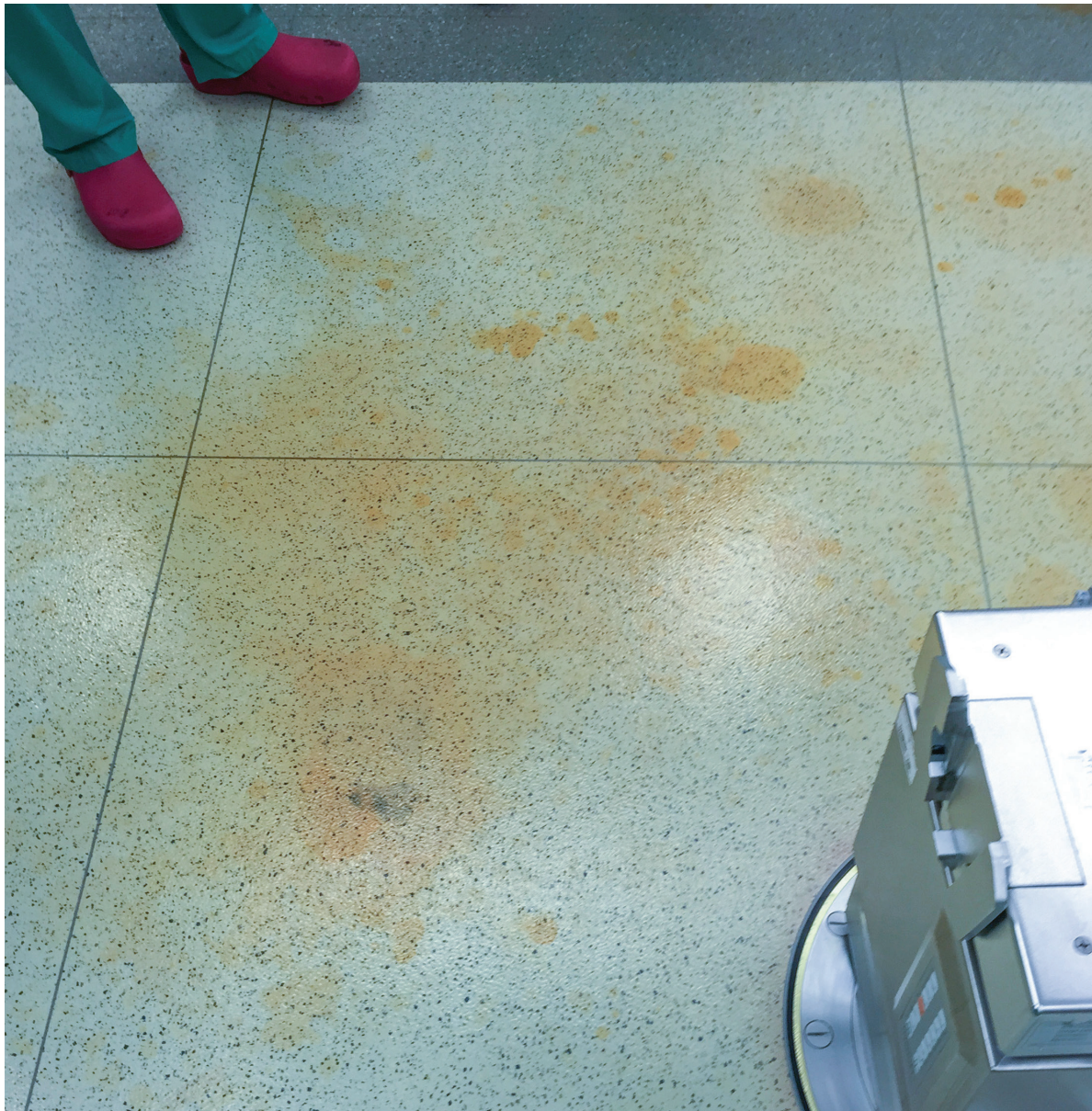
Photograph 6.5.4 A fragment of floor covering next to an operating table damaged by disinfectant agents (finishing materials should be adjusted to chemical agents applied during the procedures); photographed by the Author, 2016
