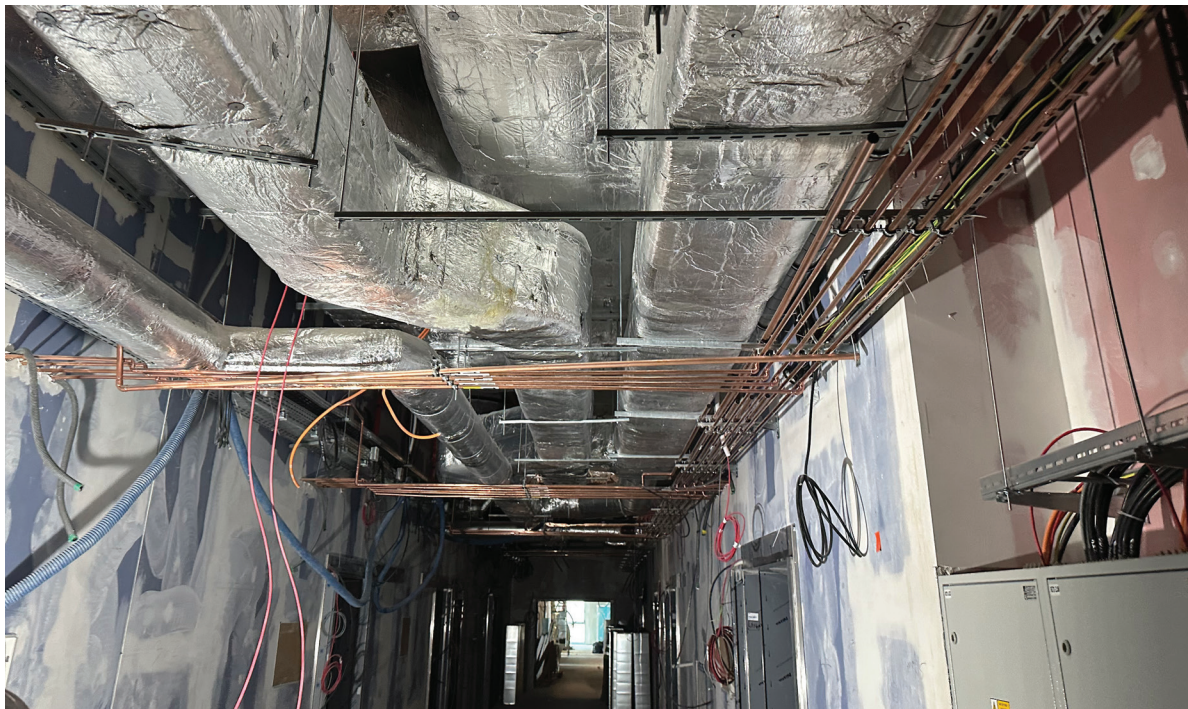
Photograph 3.1.1 A corridor (technical infrastructure in a modern hospital is an extended, complex structure that requires the HAI risk analysis); photographed by the Author, 2014
