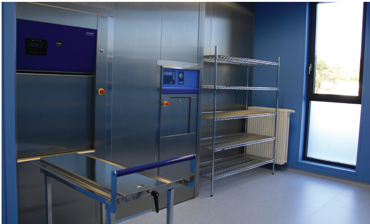
Photograph 6.4.3 A central sterilisation unit (physical separation of the dirty, clean and sterile sections allows for reducing the possibilities of secondary contamination of medical instruments); photographed by the Author 2016
