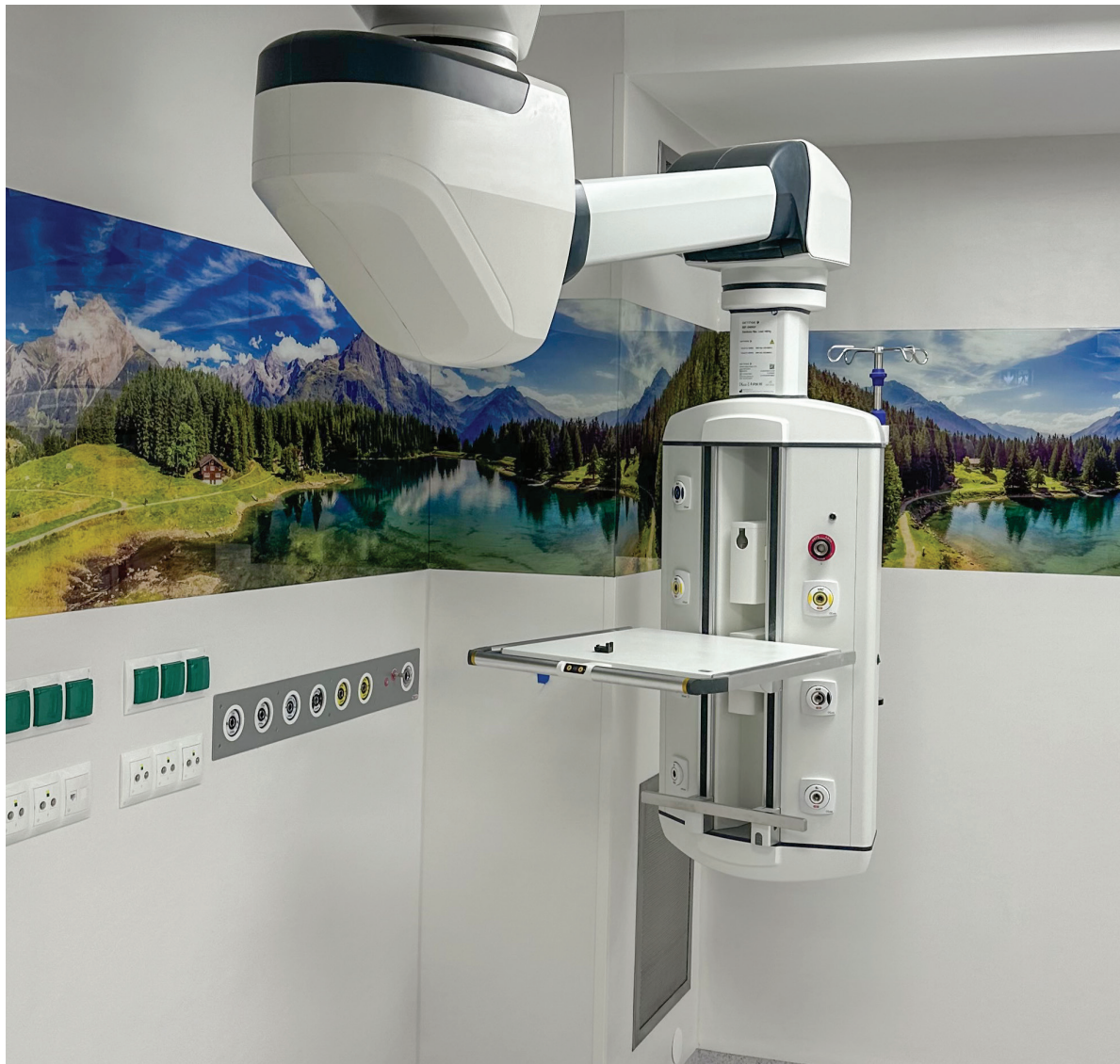
Photograph 3.3.1 The colour palette of an operating suite should allow for the possibilities of optical inspection of cleanliness; designed and photographed by the Author, 2023
