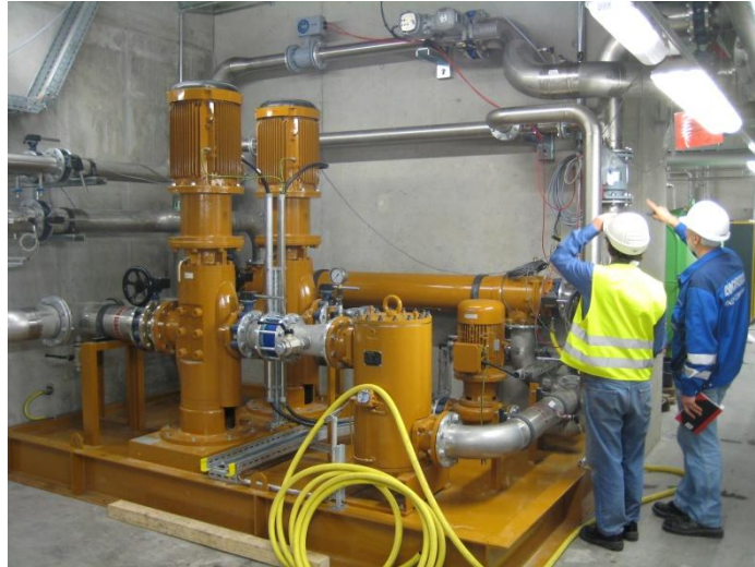
Figure 2.21. External water cooler, Kopswerk II 2 PSP power plant
