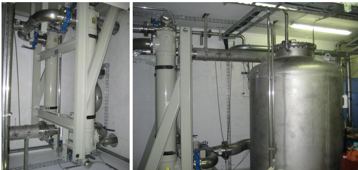
Figure 2.22. External oil tank and coolers, Feldsee PSP power plant
