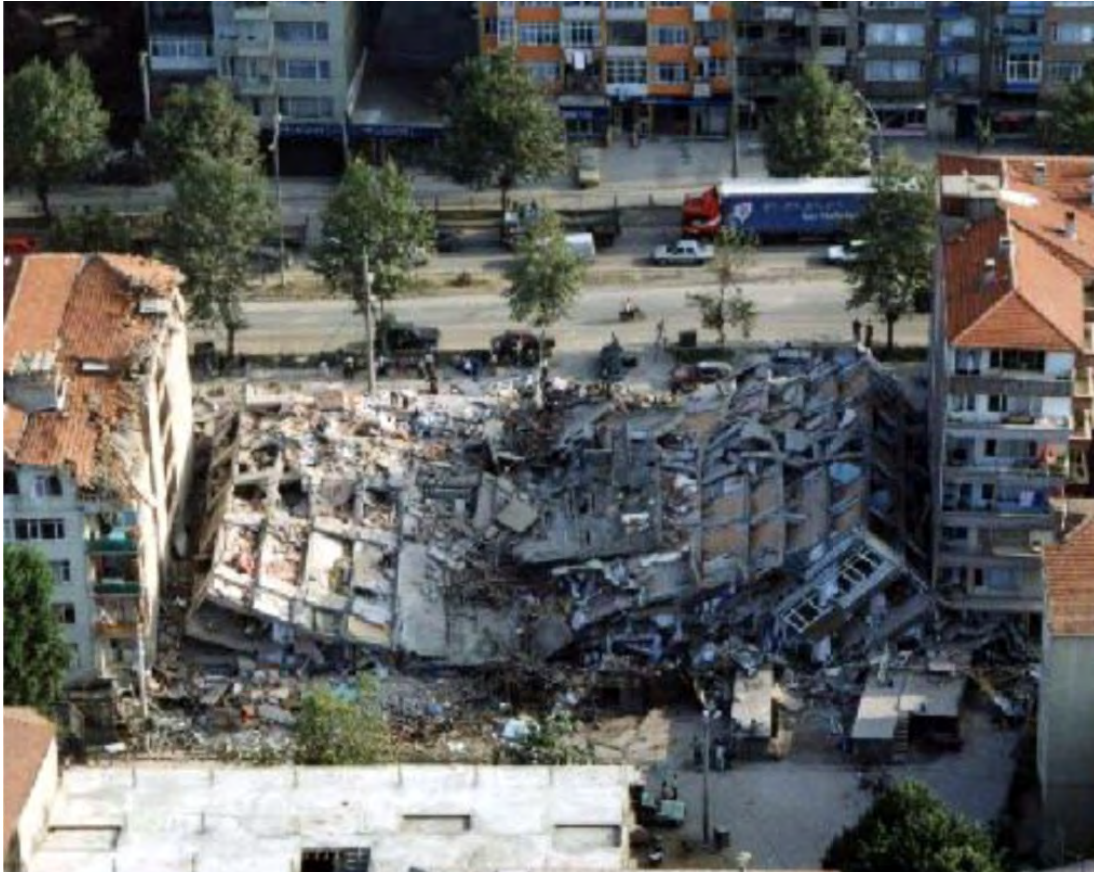
Fig. 1.4: Progressive collapse of building (Kocaeli earthquake, 1999)
