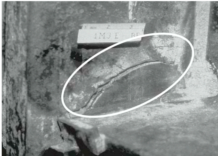
Fig. 2.3: Damage to beam-to-column connection – crack in a flange of I cross section (Naeim 2001)
