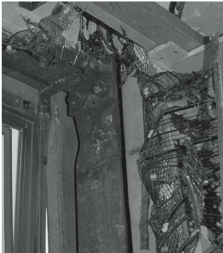
Fig. 2.4: Buckling of the top of column as the result of the 1964 Alaska earthquake (Elnashai and Di Sarno 2008)
