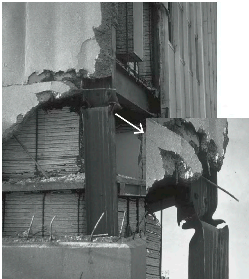
Fig. 2.6: Damage at the top of the I column as the result of the 1964 Alaska earthquake (Elnashai and Di Sarno 2008)
