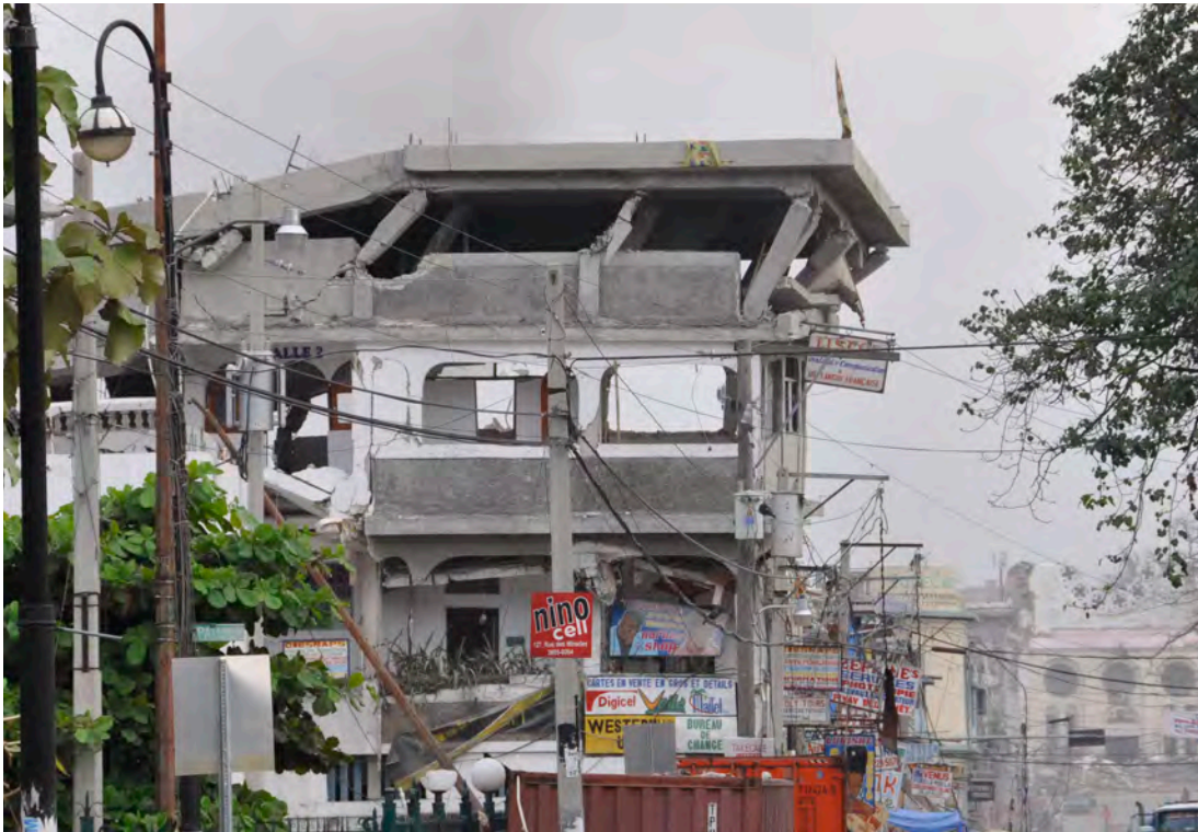
Fig. 1.3: Soft-storey failure of the top storey of building (Haiti earthquake, 2010)
