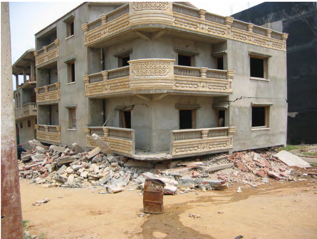
Fig. 1.1: Soft-storey failure of the first storey of building (Boumerdès earthquake, 2003)
