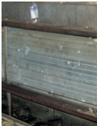
Fig. 11. Oil contamination visible on the walls of cooling chamber
