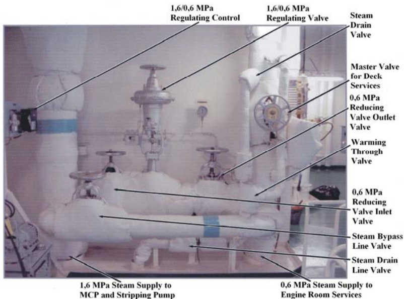
Fig. 8. Thermal isolation of valves and pipes in the steam distributor
