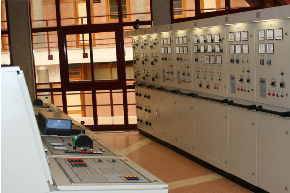
Fig. 2 MED3DH Engine Room Simulator – Switchboard panels
