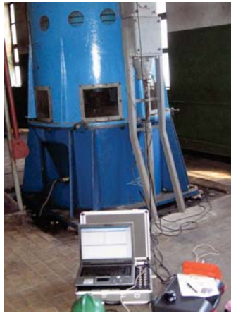
Fig.1. Electrical motor of mixed flow pump
