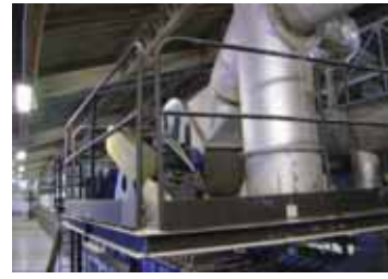
Fig. 1.3. A row of ventilators placed on a common foundation
