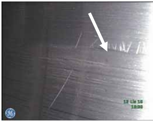
a) cylinder bearing surface - friction traces originated from the piston leading part
