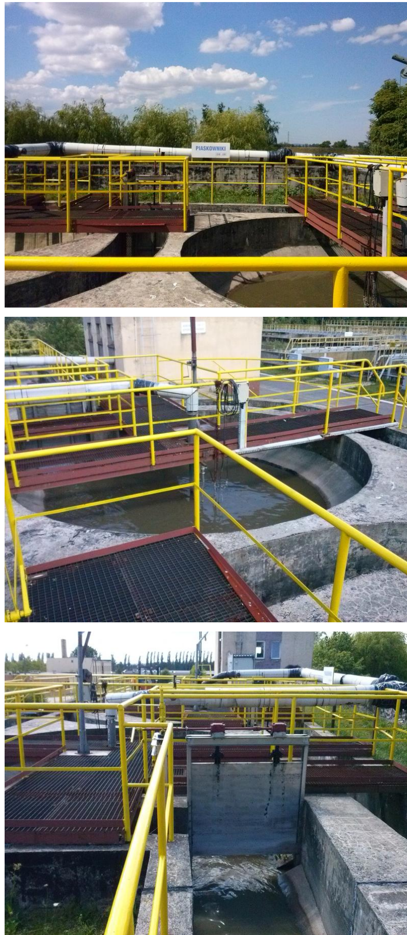
Fig. 2.7. Circular grit chambers as a part of municipal wastewater treatment plant in Tczew, Poland
