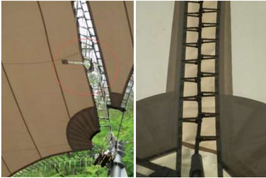
Fig. 1.12. Some of the problems with the new canopy covering: tear propagation (left) and a need to change joining shackles (right)
