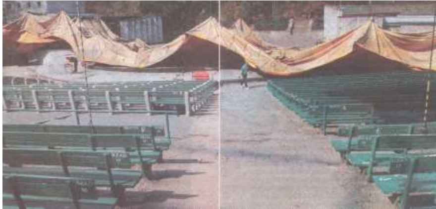
Fig. 1.10. Putting down the roofing structure of the Forest Opera in Sopot (Poland) before winter season [81]
