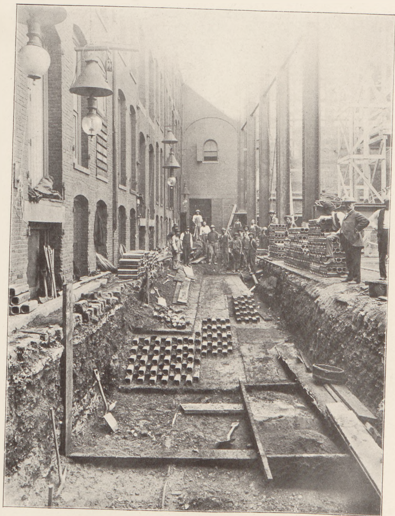
EDISON ELECTRIC ILLUMINATING CO, CONDUIT, ATLANTIC AVE., OPP. PEARL.
